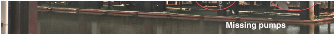
The two pumps on the right, E4 and E5, are missing from the elbows above. Pumps can be seen on the two units to the left. Click to enlarge. Photo by Danielle Bell
