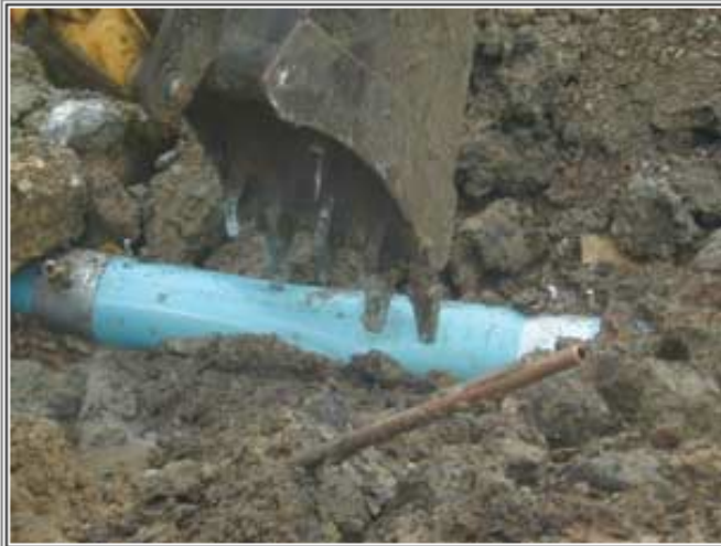
Water One put C909 plastic pipe to the test with a backhoe before putting it into use.
