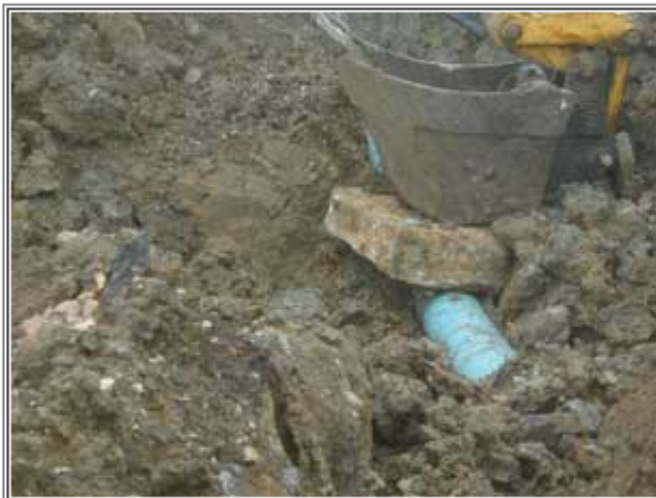
Hot soil in the Water One district calls for a pipe that won't corrode.
