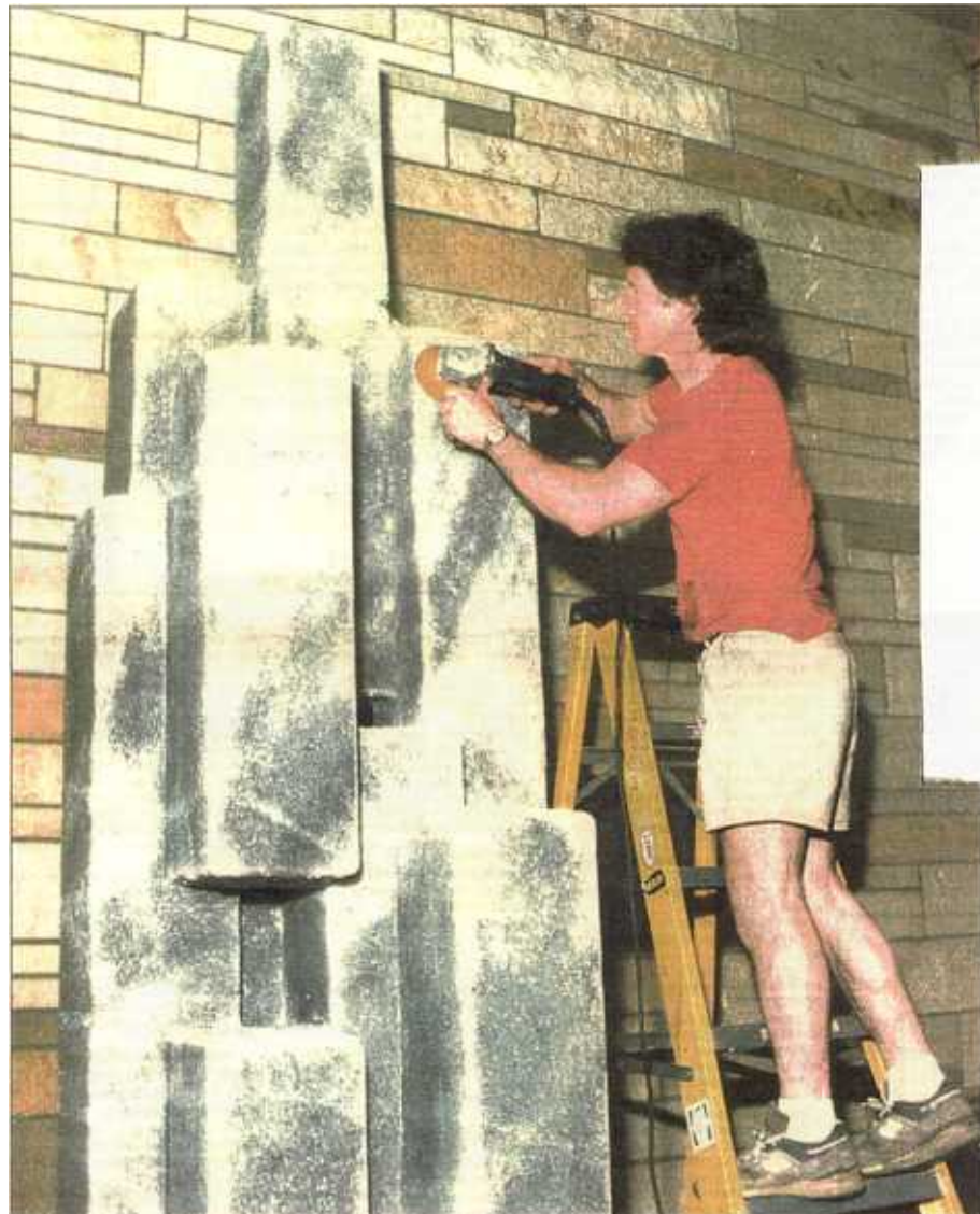
LEFT: The installation complete, Erdman still needs to doctor the piece. Moisture build-up from the salt requires a periodic sanding to remove excess salt.
