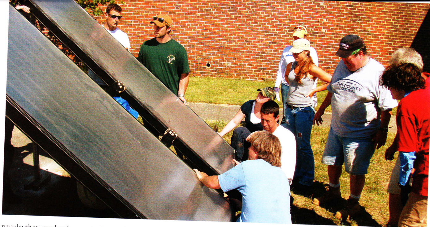
(above) CCCD students and faculty install a solar hot water panel; (below) CCCC students take pond samples for evaluation.
